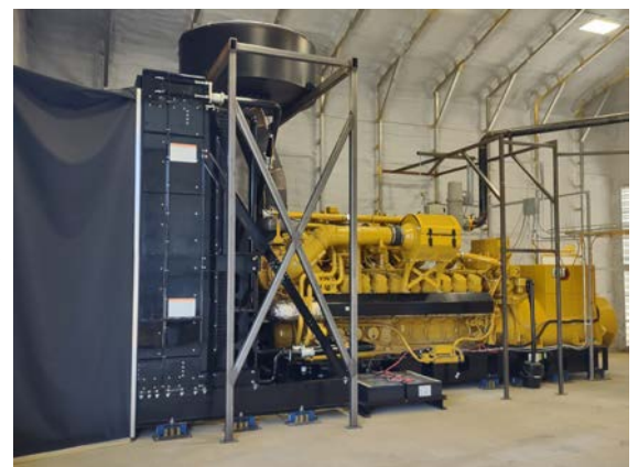
Madison Electric's Cat G3520 natural gas generator. With 2500 kw output, this device is located at the Jones Street power station.
